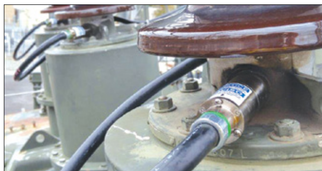
Condition monitoring of 132 kV bushing
